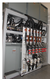
Stationary custom panel work
