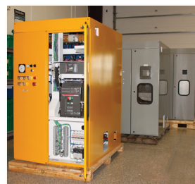
AC and DC Locomotive Traction Lockers
