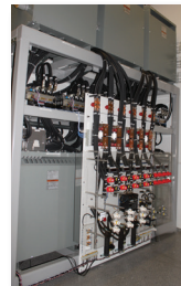
Stationary custom panel work
