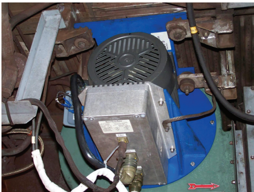
Example of Mini-VFD attached to blower motor
