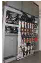
Stationary custom panel work
