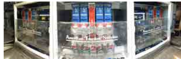
Panorama of Alcatraz Flyer engine room with three ATS racks installed. This ferry is part of the Hornblower fleet; one of the four HMS ships on which we have installed propulsion systems.
